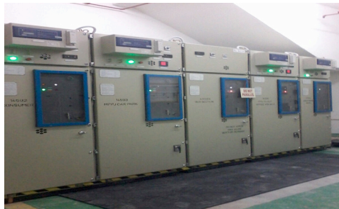
Figure 3. Installation of the magnetic actuator driven switchgear in the trial site
