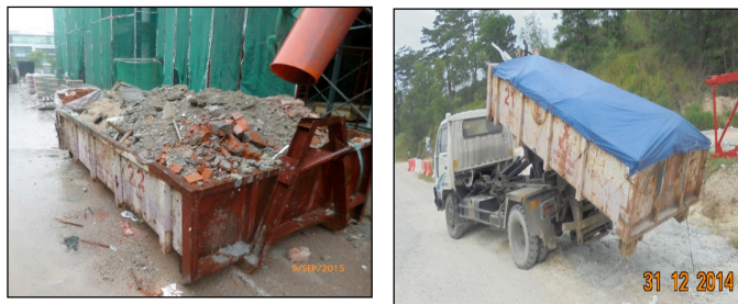
Figure 1. Concrete and masonry waste
