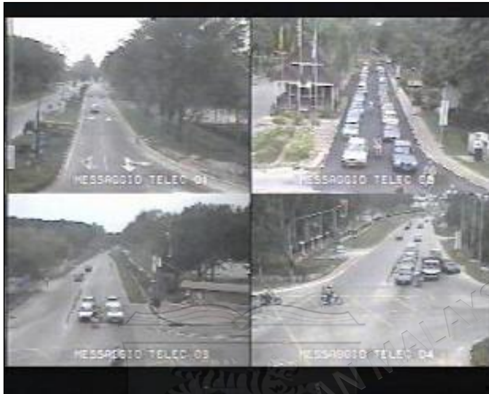
Figure B.5 Video display in control room from different traffic junction
